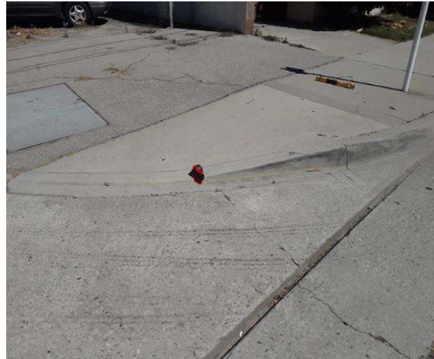
Curb Ramp , Landings And Transitions : Bottom Landing Change in Level
