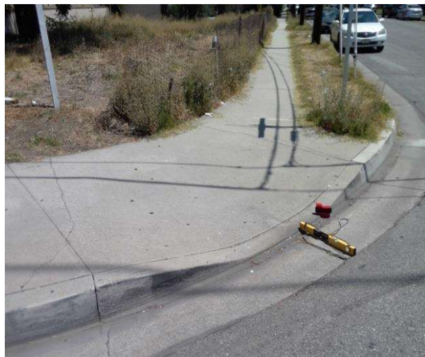
Curb Ramp , Landings And Transitions : Bottom Landing Change in Level
