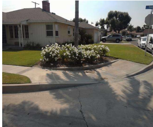
Curb Ramp , Landings and Transitions : Top Landing Right Side Clear Length - Parallel Curb Ramp
