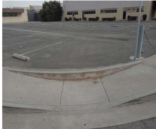
Curb Ramp , Landings and Transitions : Top Landing Right Side Slope - Parallel Curb Ramp
