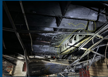
Fire compromised the structural integrity of the framing members
