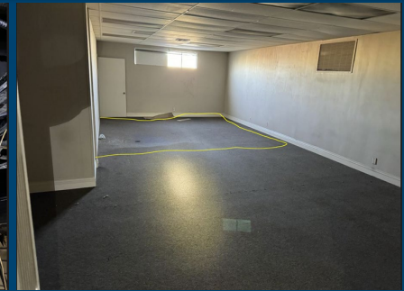
2 nd floor has begun to sag due to damaged floor joists and framing members
