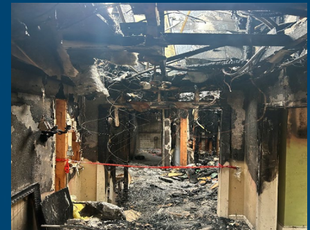
Fire compromised the structural integrity of the 2 nd floor and roof
