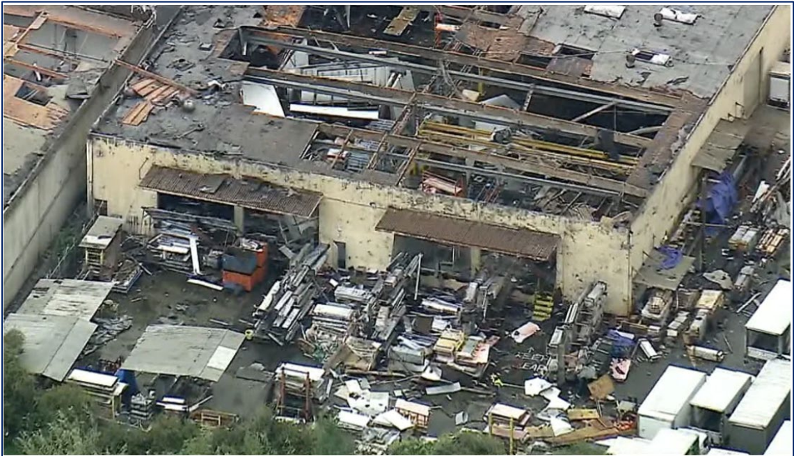
Figure 3.27: EF1 Tornado rips off Roof of a building in Montebello, March 22, 2023
