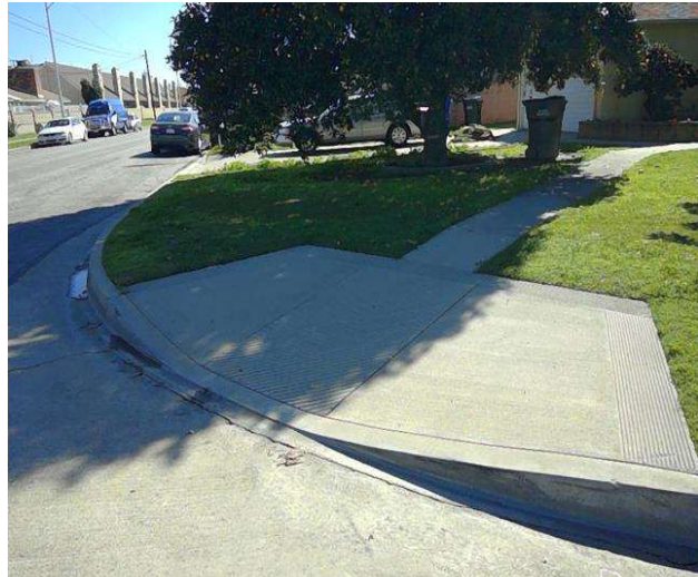
Curb Ramp , Landings and Transitions : Bottom Landing Change in Level - Curb Ramps
