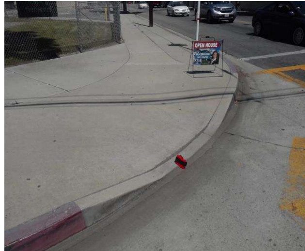
Curb Ramp , Landings and Transitions : Bottom Landing Change in Level - Curb Ramps
